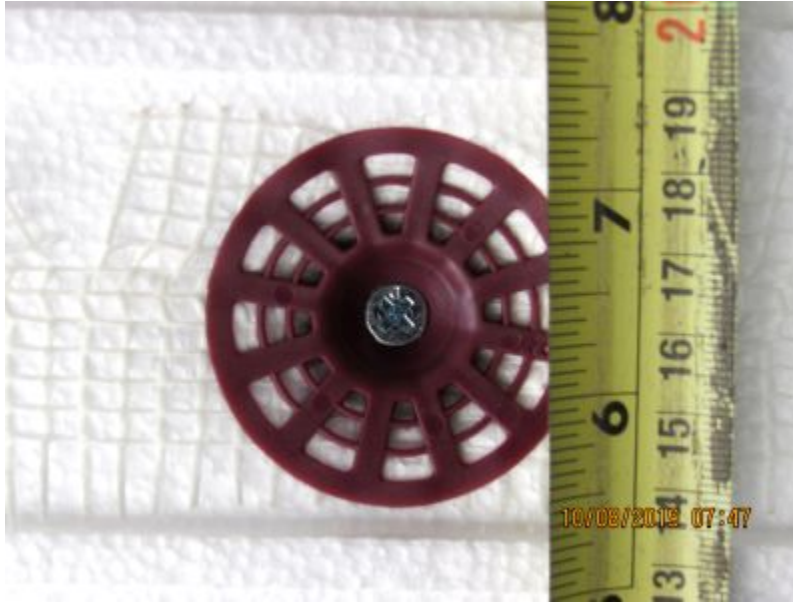
Photo No. 9 Fastener Heads With Mesh
