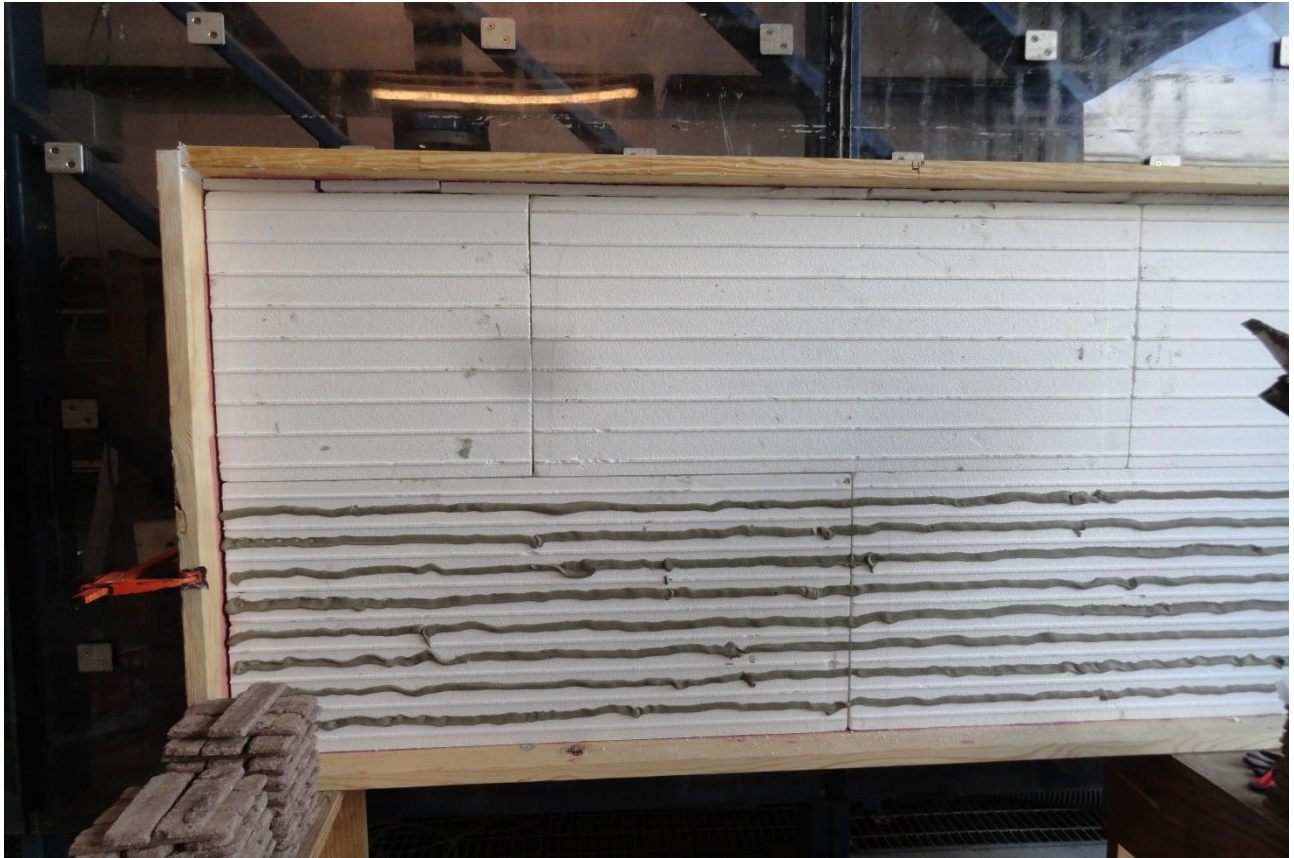
THIN BRICK INSTALLED INTO HORIZONTAL 3/4" BEAD OF OLD MILL BRICK & PANEL ADHESIVE
